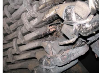
Photo 2. Several inches of copper burned away on a stator bar.
