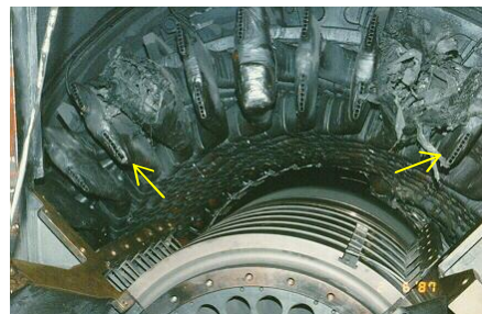
Photo 13. Ring-of-fire failure of a stator endwinding. Arrows identify typical exposed bare conductor locations.
