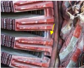
Photo 18. Minor iron discoloration judged to be insignificant.
