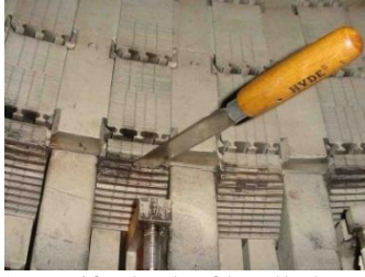
Photo 17. Knife check of locally loose core.
