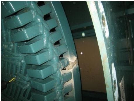
Photo 5. Dust generation from failed dry tie.
