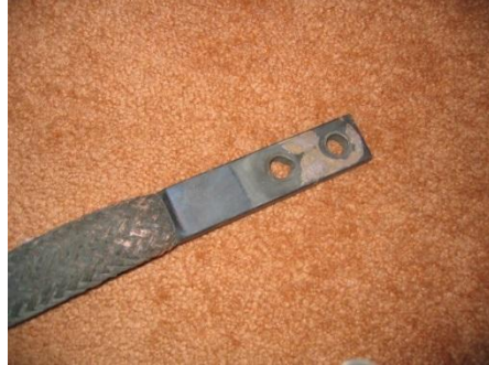
Photo 7. Failing flexible lead, high voltage bushing to isophase bus.
