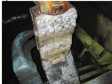
Photo 8. Bolted high current connection.
