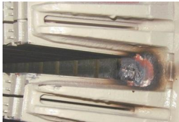
Photo 19. Same core location after a few hours of excitation.
