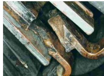
Photo 12. Phase-to-phase copper burning due to non-mica connection insulation failure.
