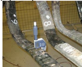
Photo 16. Remaining groundwall measured 20% of original thickness.
